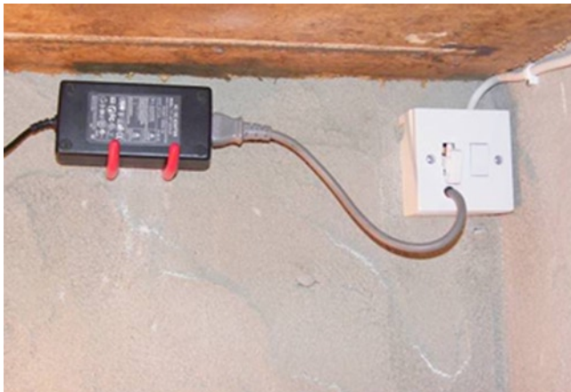
Figure 11-11. The 12V DC power supply
